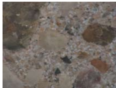
Fig. 3. Surface of concrete sample (1) after 50 days experiment duration (magnifications 20×4.5)
